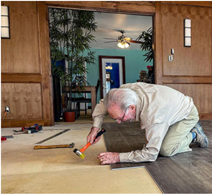
Uncle Bob finished installing flooring in the Clubhouse. Note the new wood paneling.
